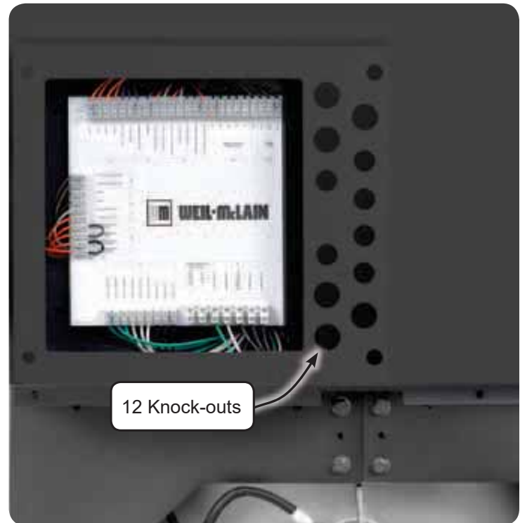
Figure 50 Wiring entrances in terminal box rear of boiler
