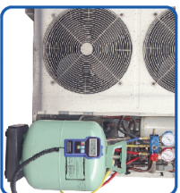
Charging for A/C System
